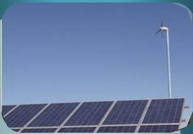
Wind turbine and solar panel installation at the COSSA school facility in Wilder, Idaho.
