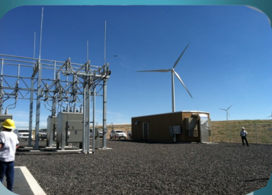
Horse Butte Wind Project site 15 miles east of Idaho Falls near Kepp's Crossing.
